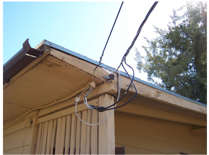
Main overhead power
