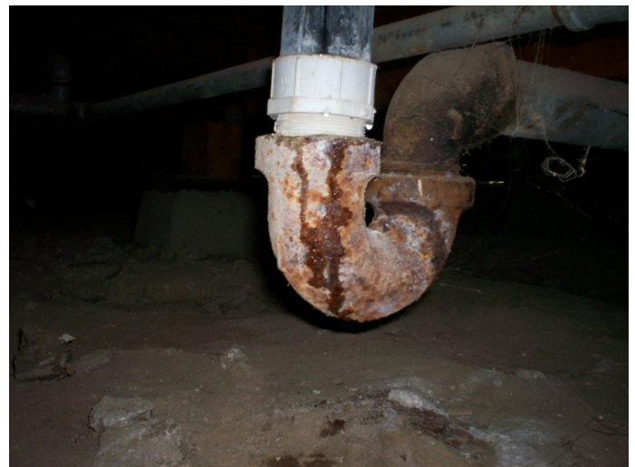
Plumbing in Crawlspace
